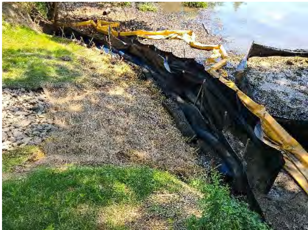
Fig 2: Temporary BMPs installed at toe of slope and intertidal zone at Gundalow landing/east side of the Bay. Viewing south. (07-02-20).
