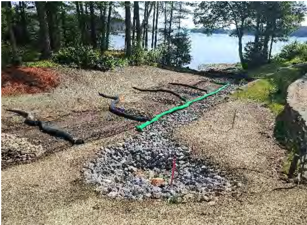
Fig 4: Drainage culvert & riprap swale-temporary BMPs installed on slope above manhole at Gundalow landing/east side of the Bay. Viewing south. (07-02-20).
