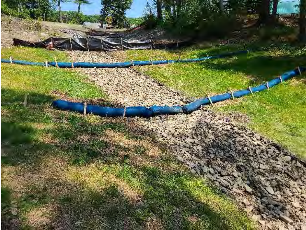
Fig 3: Temporary 6 inch stone installed in place of the small diameter gravel on path at Gundalow landing/east side of the Bay. Viewing east. (07-02-20).
